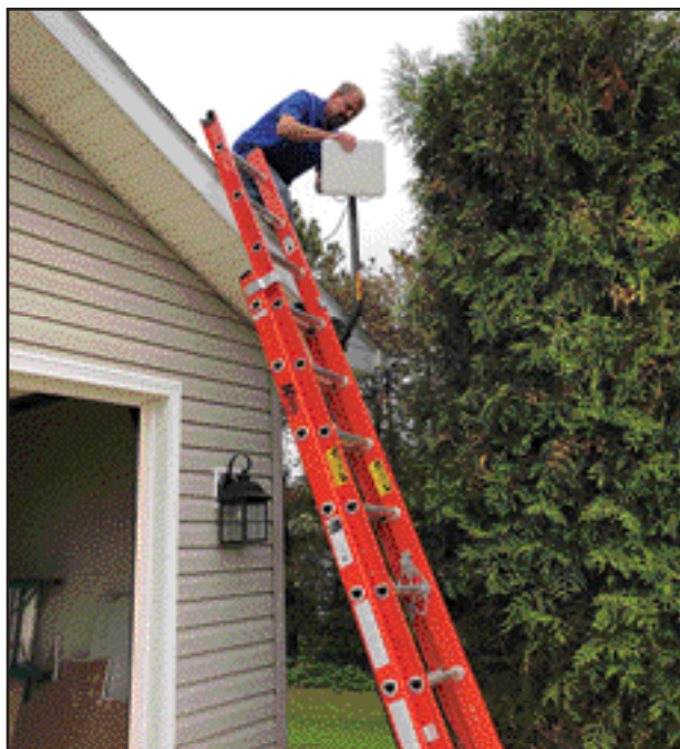
VIBRANT installer Scott Ernst installing one of the first fixed wireless services this summer.
